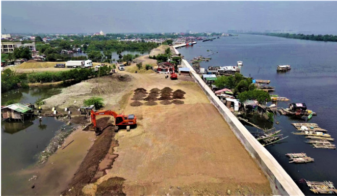
Ongoing construction activities in Bacoor Diversion Road Project. Photo by: DPWH Region IV-A
