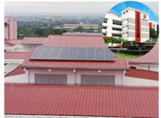
Five Storey Student Services Center II Capacity 10KVA
