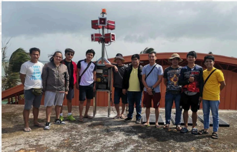
The SIGAW Project Team together with Mr. Nel B. Resplandor, Calauag MDRRMO and his staff after the SIGAW Calauag Unit installation
