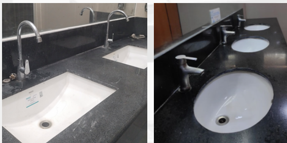
WATER-EFFICIENT FAUCET INSTALLED IN COMFORT ROOMS
