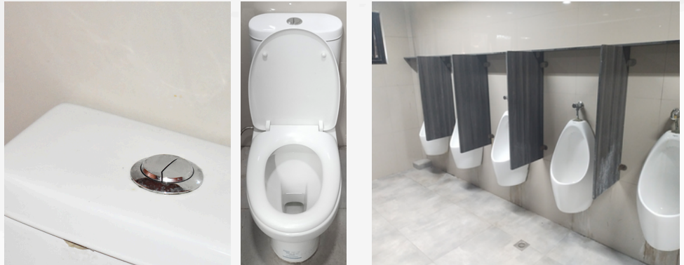
WATER-EFFICIENT WATER CLOSET FLUSH TANKS WERE INSTALLED IN COMFORT ROOMS WITHIN THE UNIVERSITY
